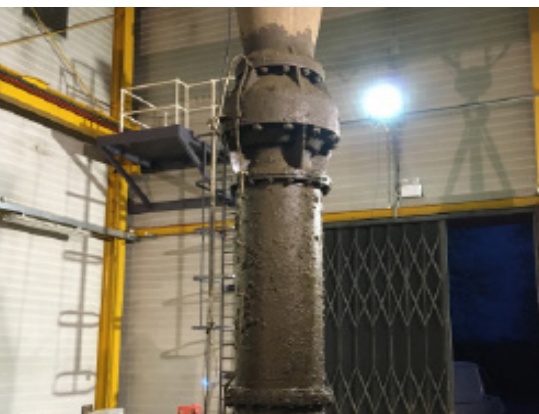
Old river intake pump ins-itu
