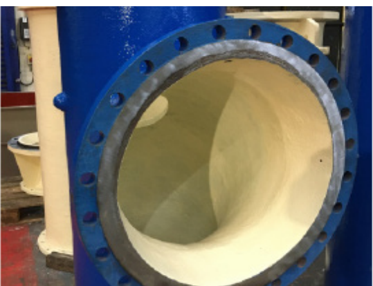
Refurbished pipework with WRAS-approved coating
